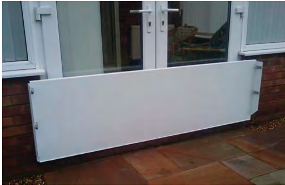
Right: Flood barrier gates installed at doorways before a flood event is a form of dry floodproofing. Image courtesy of New York City Planning Department.
