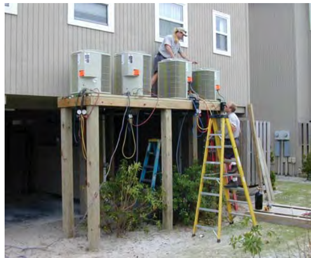
Two workers are elevating condenser units on a platform above the Base Flood Elevation. Image courtesy of FEMA.
