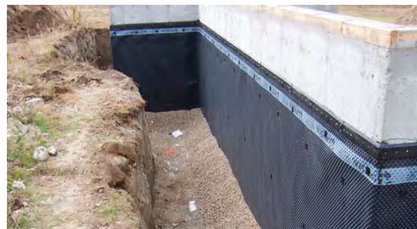
A waterproofing membrane is installed below grade to prohibit the flow of water into basement areas. Image courtesy of Foundation King.
