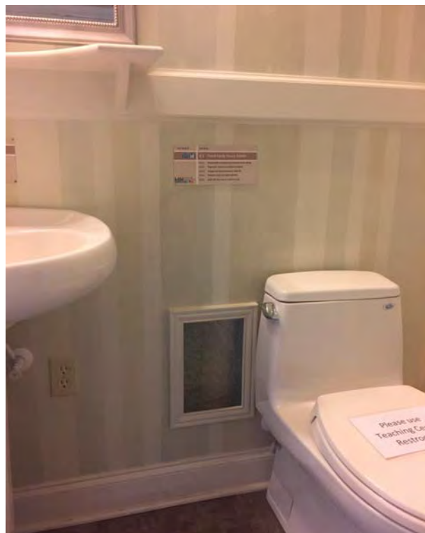
View of the plywood wainscoting in the LaHouse bathroom which has been painted to match the upper portion of the wall which is sheathed in drywall. Image courtesy of Gulf Coast Community Design Studio.
