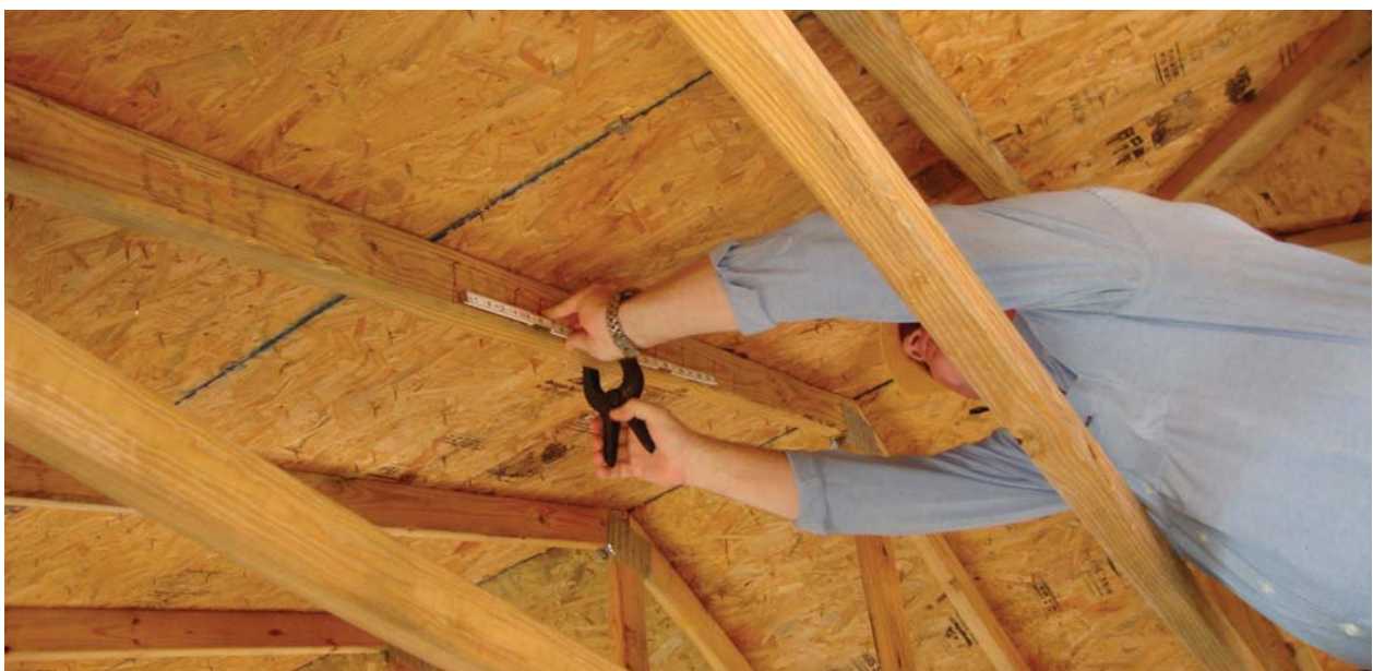
Figure 1. FORTIFIED Home™ inspector checks nailing pattern in roof sheathing. Image courtesy of Habitat for Humanity of the Mississippi Gulf Coast.
