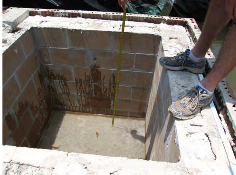
Fig. 4.37. PHOTO: Water seeping into test pod B2: cavity wall filled block, flood sim. 2.
