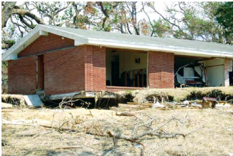
Fig. 2.9. PHOTO: Damage as a result of localized scour. (FEMA 549 2006)
