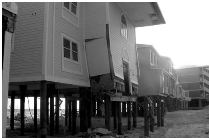
Fig. 2.6. PHOTO: Damage as a result of non-breakaway stair design. (FEMA TB-5 2008)
