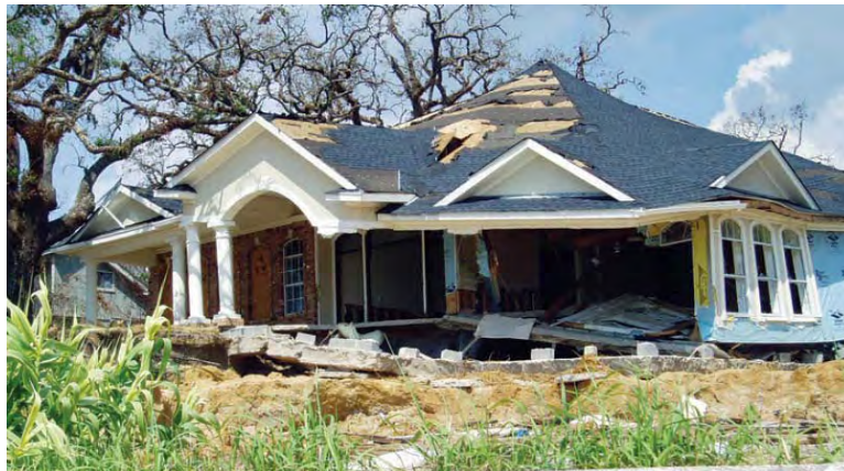
Fig. 2.4. PHOTO: Failure due to hydrodynamic forces. (FEMA 549 2006)
