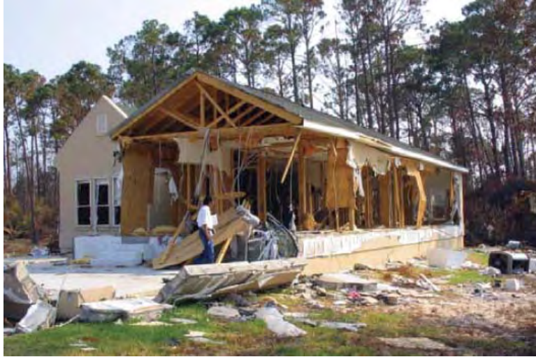
Fig. 2.8. PHOTO: Damage as a result of breaking waves. (FEMA 490 2005)
